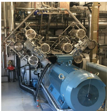
Figure 1. Heat pump installed on site.
